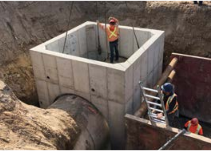
Doghouse structure in final resting position.
